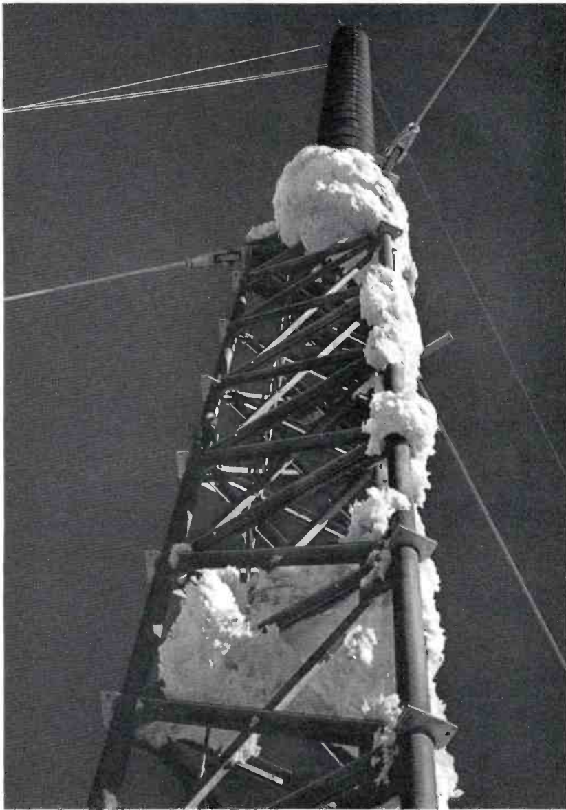
FIG. 2. A close up of the Traveling Wave Antenna. Note top guy arrangement required to support the tower and antenna against extremely high winds. Contrast, ice accumulation on tower with complete freedom from ice on antenna enclosure. This is typical.
