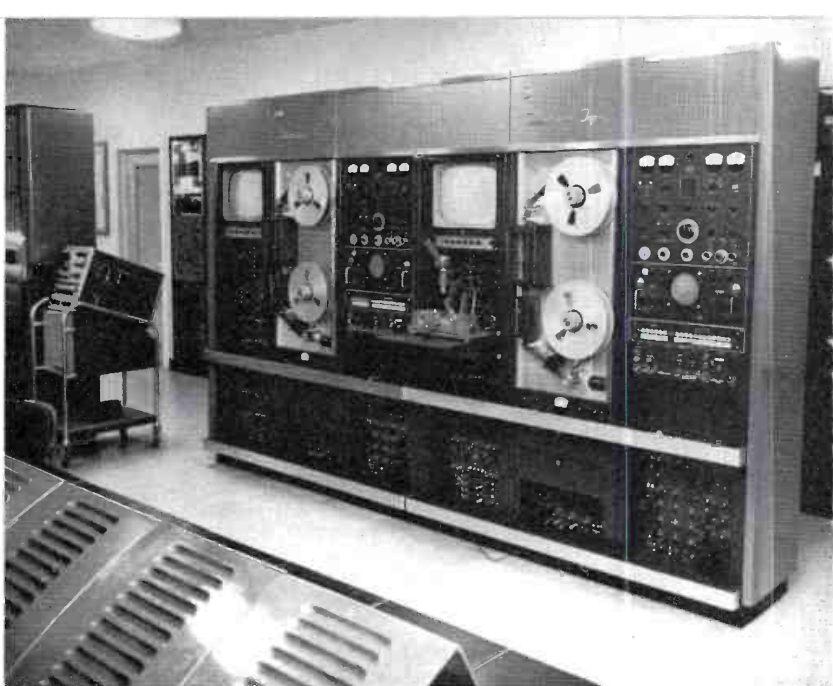
FIG. 20. Two RCA TRT-1B TV Tape Recorders, recently installed in Master Control area.
